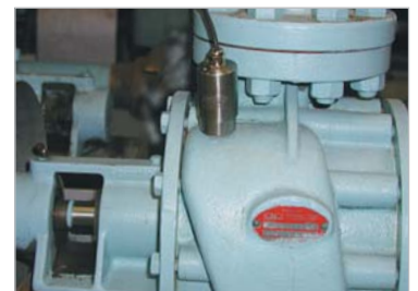
Monitor cavitation, bearings, and valves
